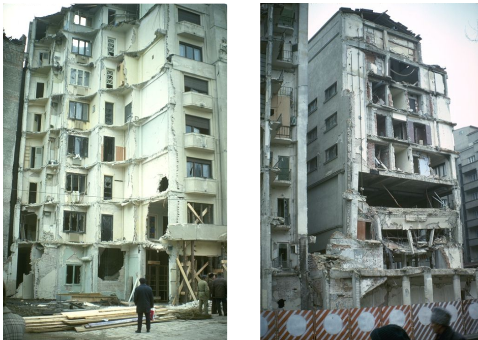
Figure 1: Pre-1940s medium and high-rise buildings that partially collapsed during the earthquake on March 4, 1977 ( http://nisee.berkeley.edu )
